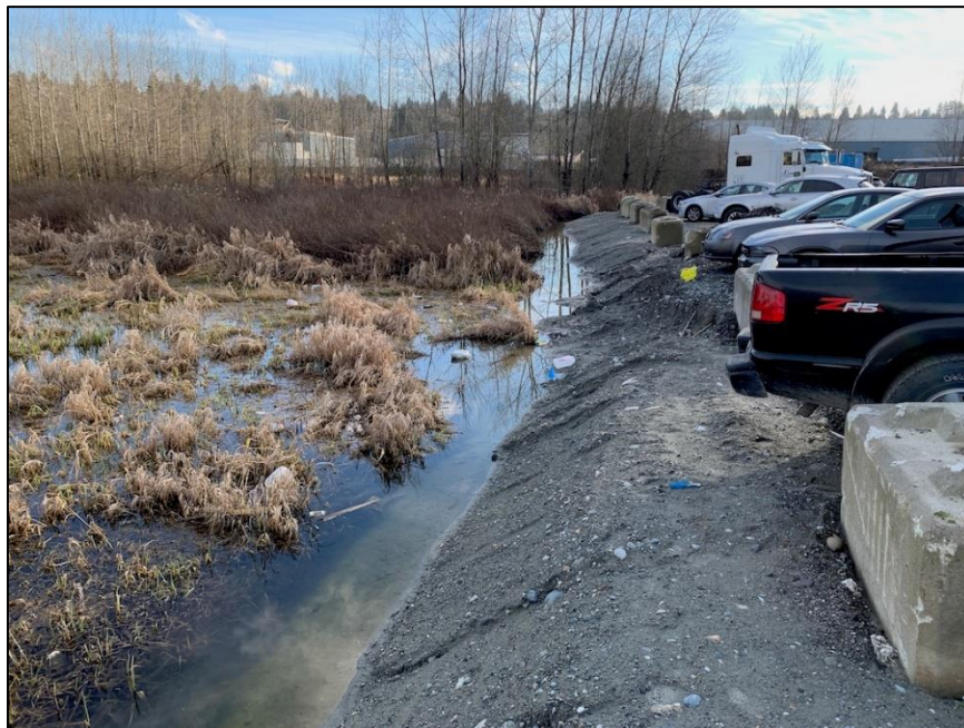
Photograph 22: South view of the west bank of Wetland D. Note the rill erosion of the fine fill material depositing sediment into the wetland. Photograph taken January 19, 2021.
