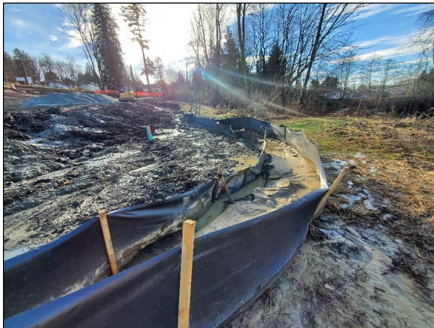
Photograph 10. Southward view of the conditions east of Wetland A where a residential development is under construction. Photograph taken January 19, 2021. The silt fences are intended to prevent further sediment from entering the wetland as shown in Photograph 8.
