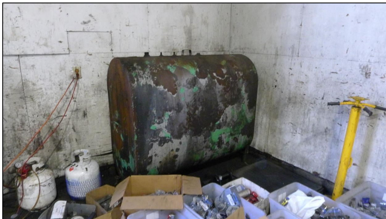
Photograph 4: Dis-used waste oil AST inside trailer repair shop at 10582 Scott Road
